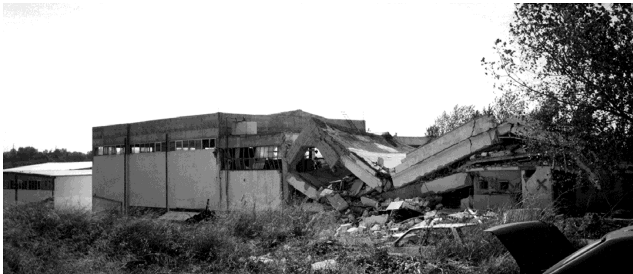
Fig. 4. Collapse of a reinforced-concrete factory in the region of Aharnes (large ellipse in Fig. 3).
