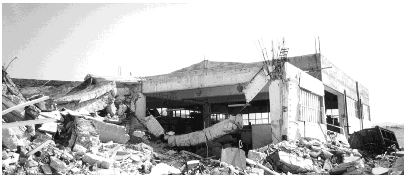
Fig. 5. Collapse of a reinforced-concrete factory located next to that shown in Fig. 4.
