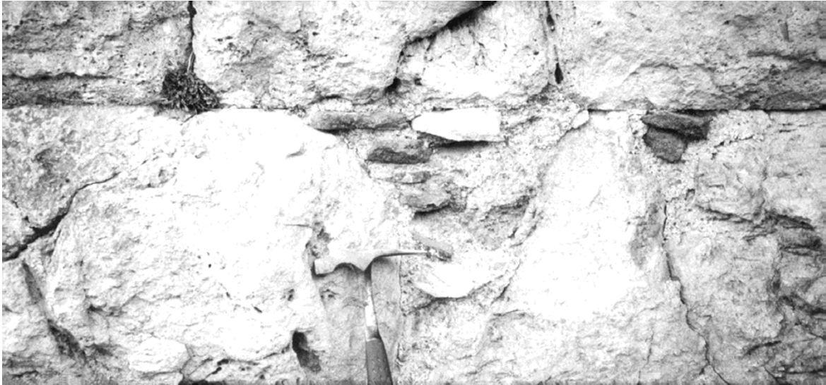
Fig. 6. Old reparation works in broken wall-stones in the Fili Fort. Reparation consists of bricks soldered by mortar.
